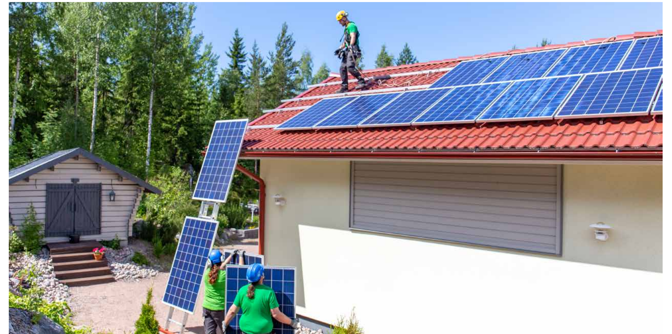
Solar power is a compelling option at the moment. The Caruna Marketplace is a great way to find suppliers of solar panels.
